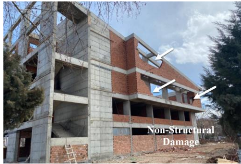
Fig 5. Building A-1 right after the 06 FEB 2023 earthquakes (37.79198°N, 37.64886°E)
