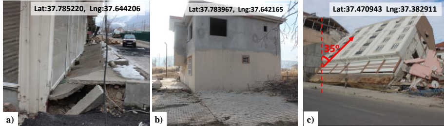
Fig 3. (a) Lateral spreading and excessive settlement, (b) punching failure, and (c) overturning of buildings in Gölbaşı
