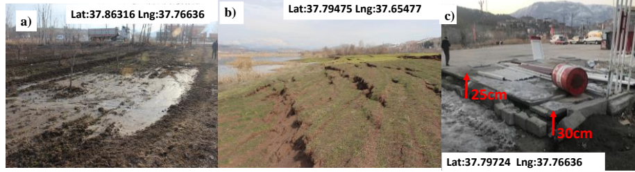
Fig 2. Some of the seismic liquefaction symptoms (a) sand/silt volcanoes, (b) lateral spreading near the Golbasi Lake, and (c) fuel tank uplift in Gölbaşı City Center
