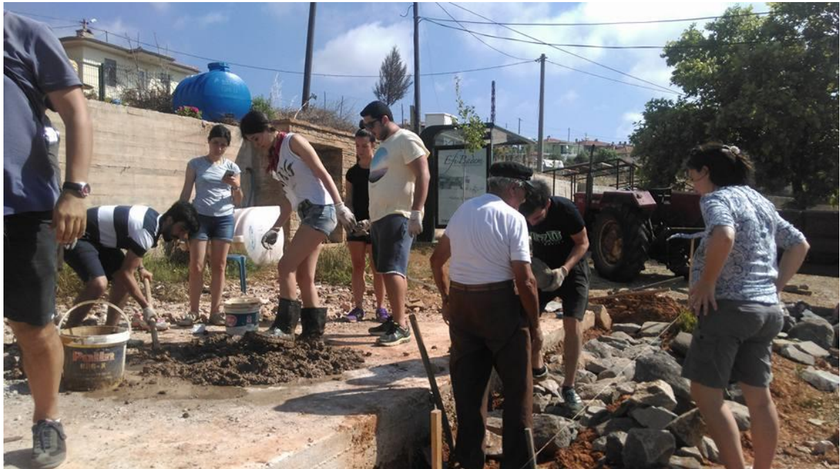
Figure 6. Regeneration of Environment workshop students and tutors bonding the traditional stone wall in Eşelek (2016).
